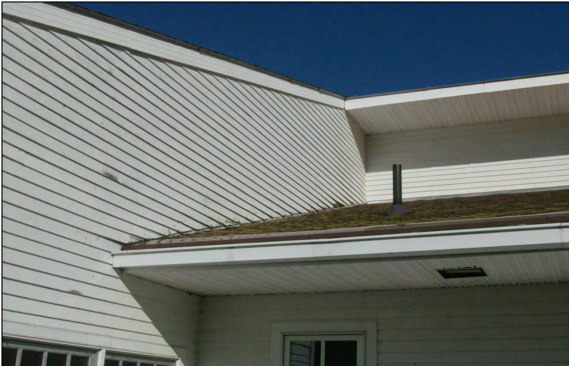
Roof at courtyard. Note rotted siding along slope of roof.
