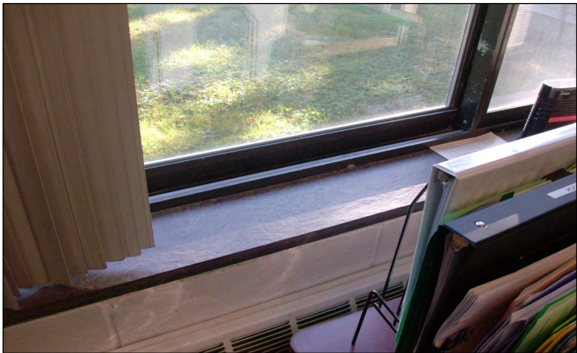
Typical casement type metal windows in 1970's wing in need of replacement.
