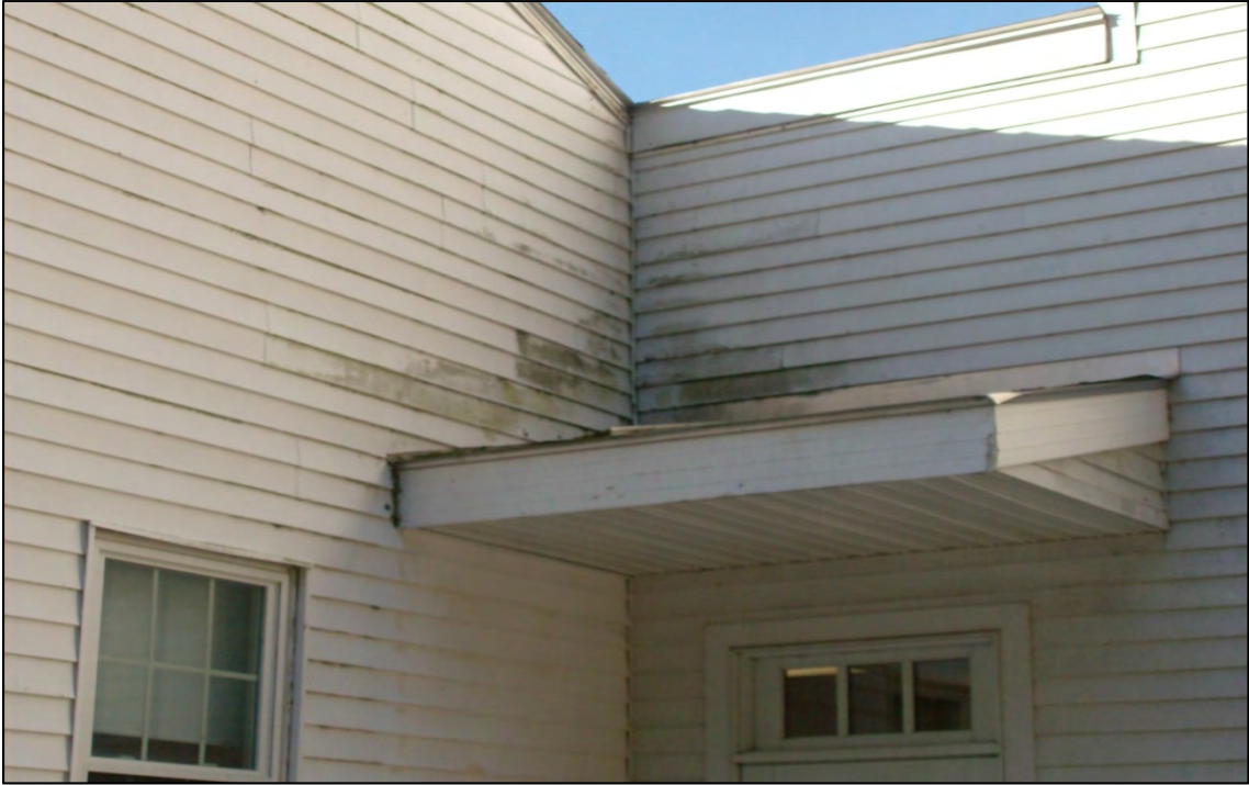
Canopy over door on east side. Note mildew and rotted siding.
