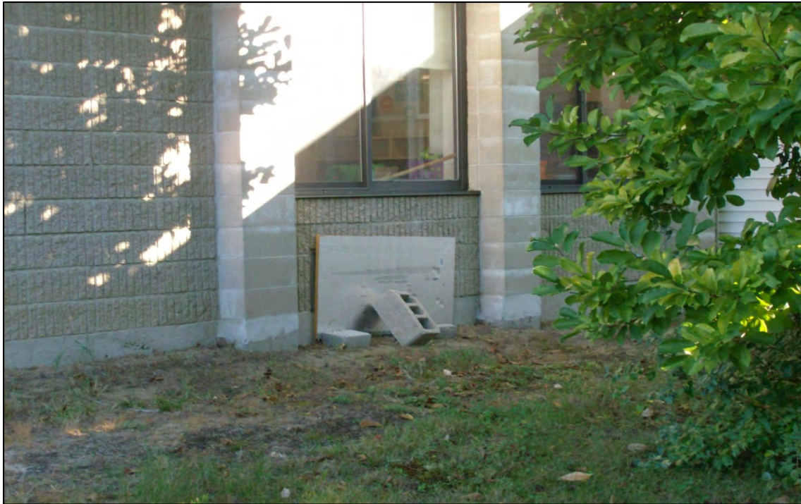
Unit ventilator grille blocked with foam panel.
