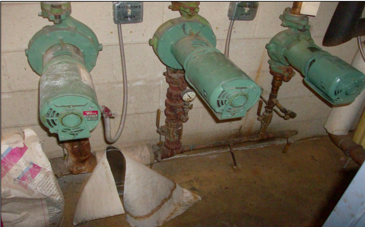
Hot water circulating pumps.
