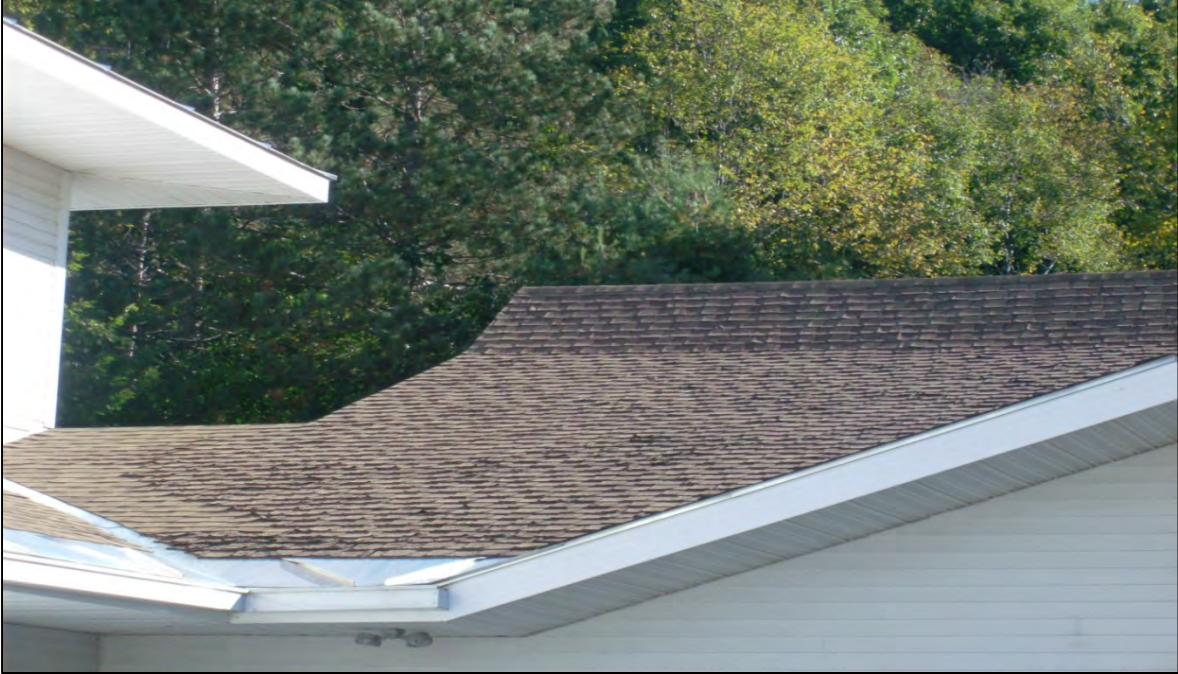
Poor condition of roof shingles on west side near courtyard.
