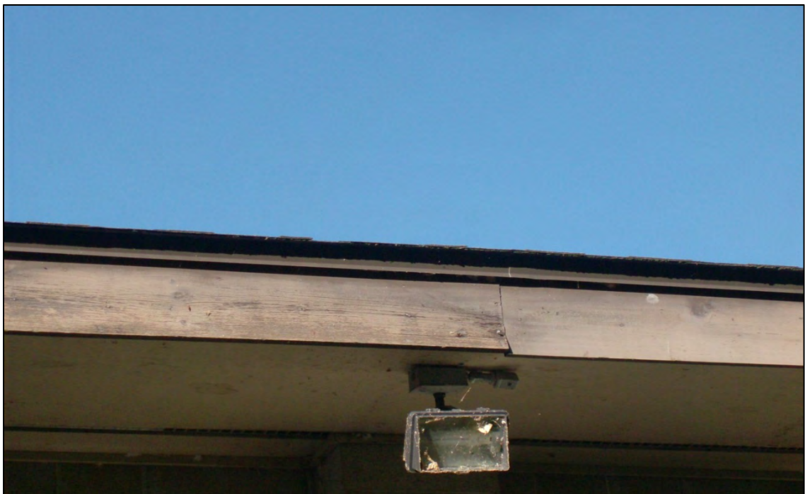
Fascia board on 1970's wing needs paint or break metal covering.
