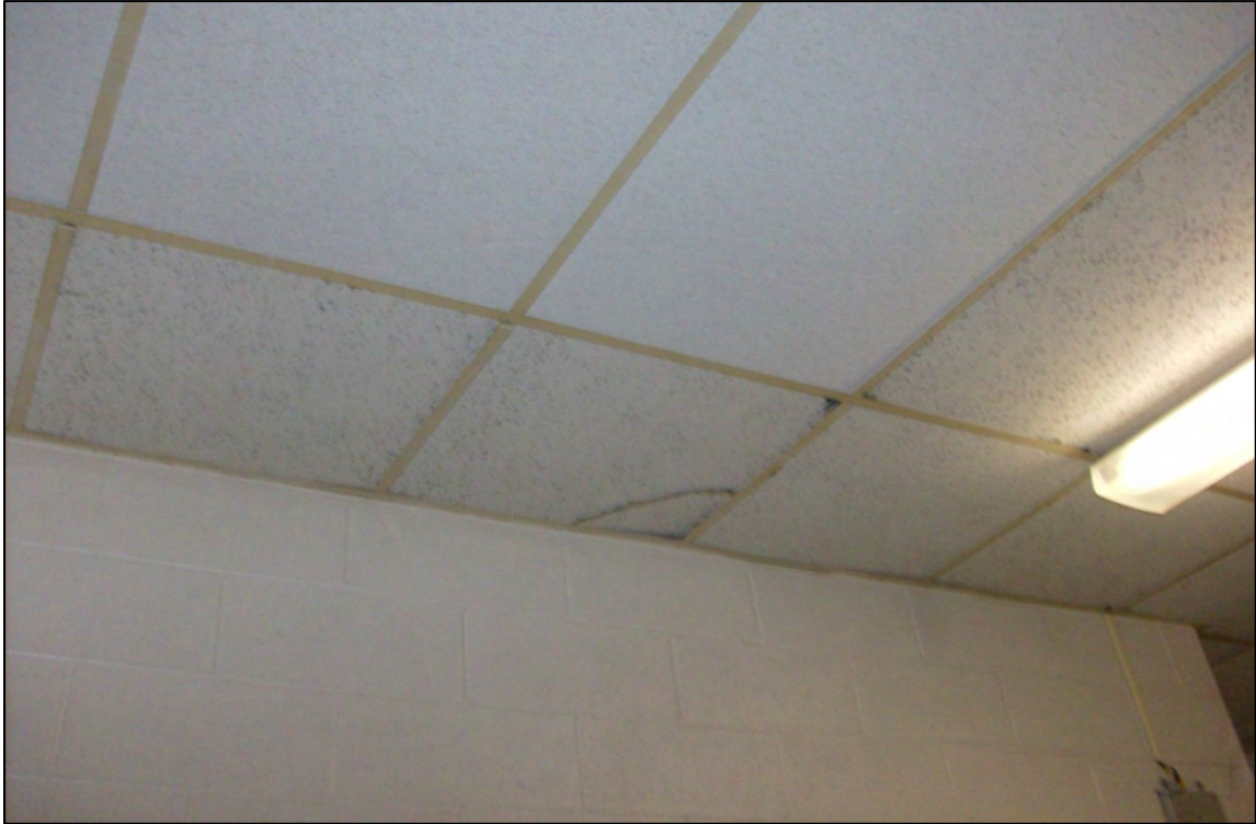
Discolored and cracked ceiling tile, typical in many locations.
