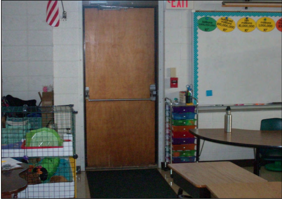
One of two doors that leak during driving rains.
