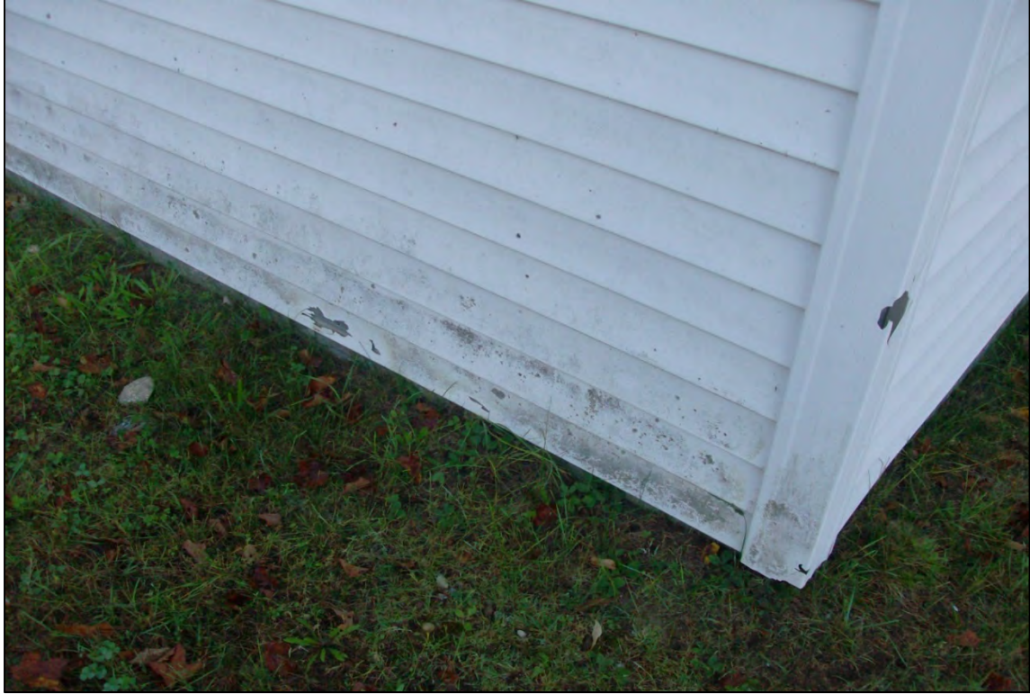
Mold growth on vinyl siding. Damage from “weed whacker”.
