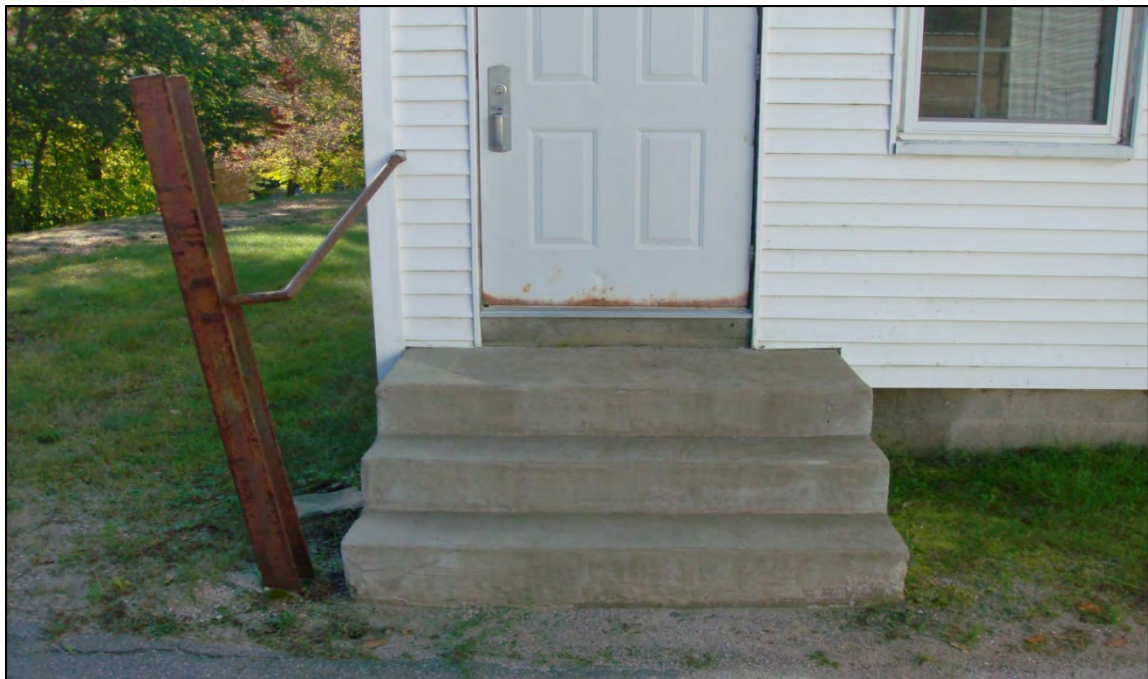
Door at Music Room. Door needs painting and railing should be replaced.
