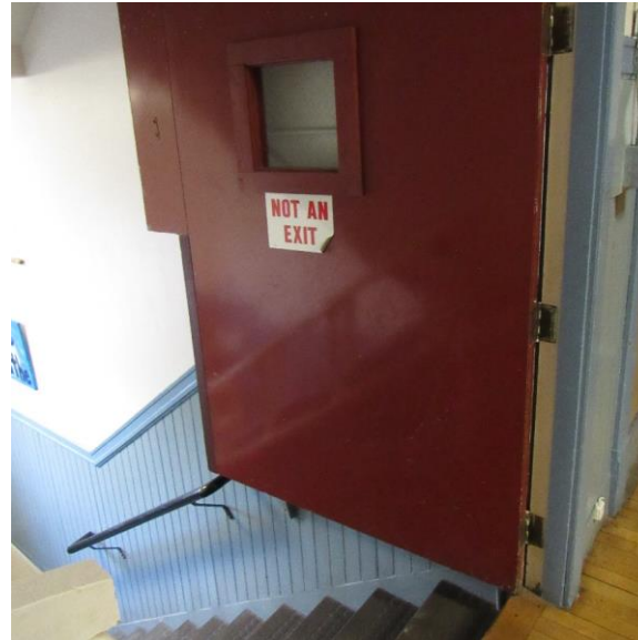
Compromised Fire Door
