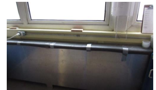
Corridor Heating Element with Foam Protection
