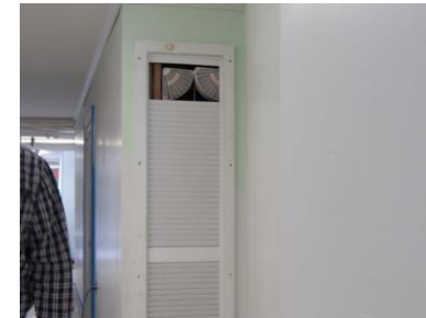
Unprotected Corridor Opening
