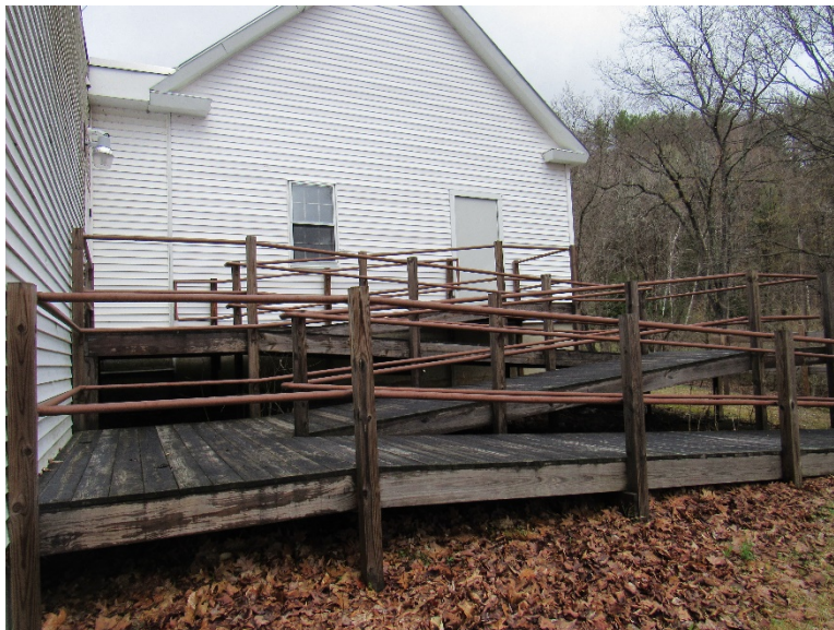
View of extensive network of ramps used as an exit discharge. Note the lack of guardrails from the higher levels.
