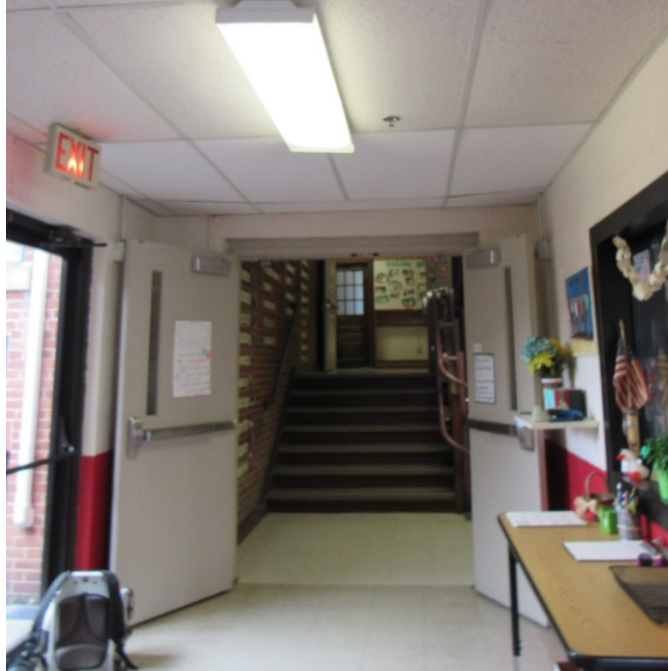
View of front lobby looking upstairs to principal's office. The lobby is open to the corridors of later wings and not fire rated nor secure.
