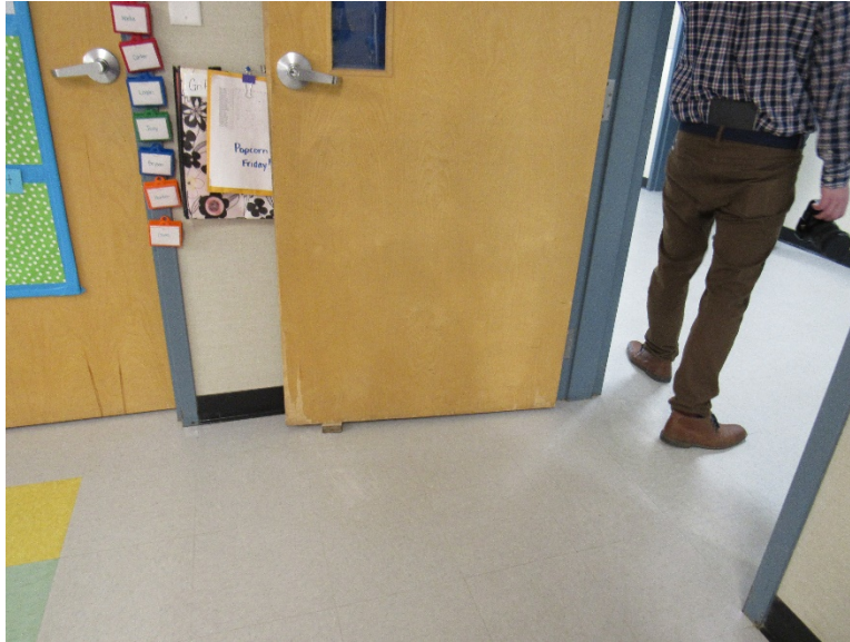
This school is mostly upgraded but some areas still show signs of wear such as this door that has been damaged by a door chock.
