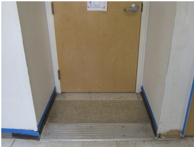
A classroom doorway that is not handicap accessible due to lack of pull-side clearance.
