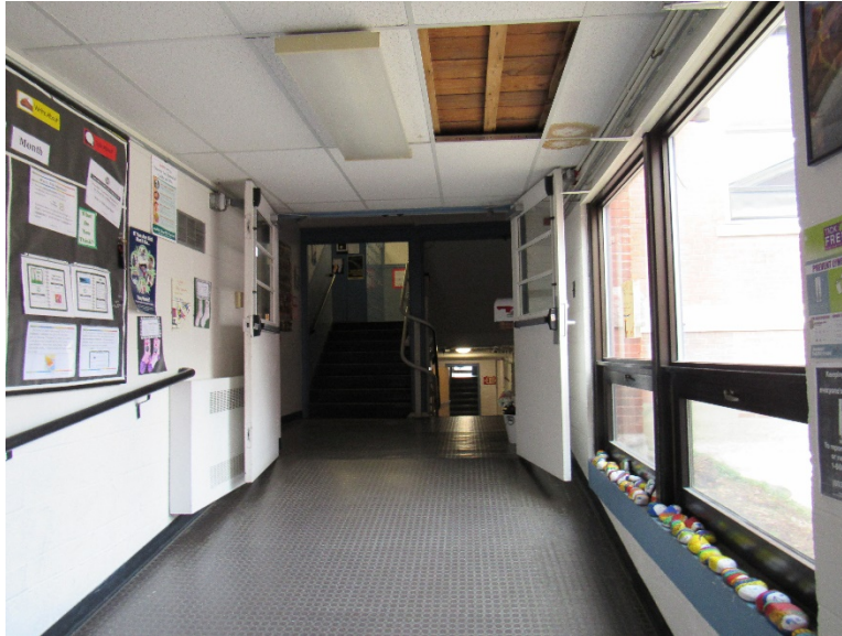
View from lobby to stairs. Note that the fire doors open onto the ramp. Also note the stair lift attached to the railing impeding with the railing use.
