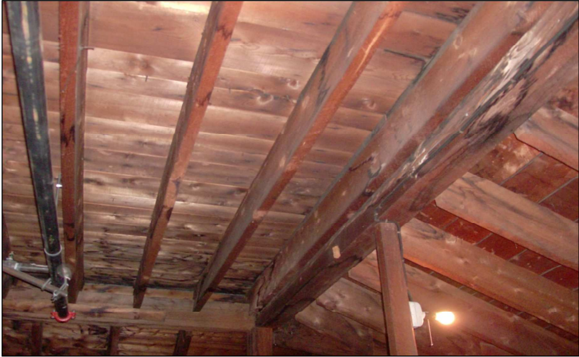
Typical wood framing in the attic. Wood staining may indicate past leakage.
