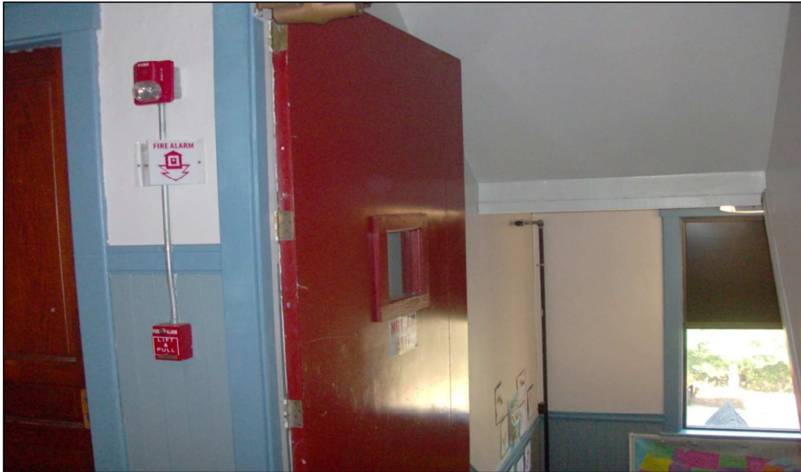
Large heavy fire door at top of stairwell in original section of building.
