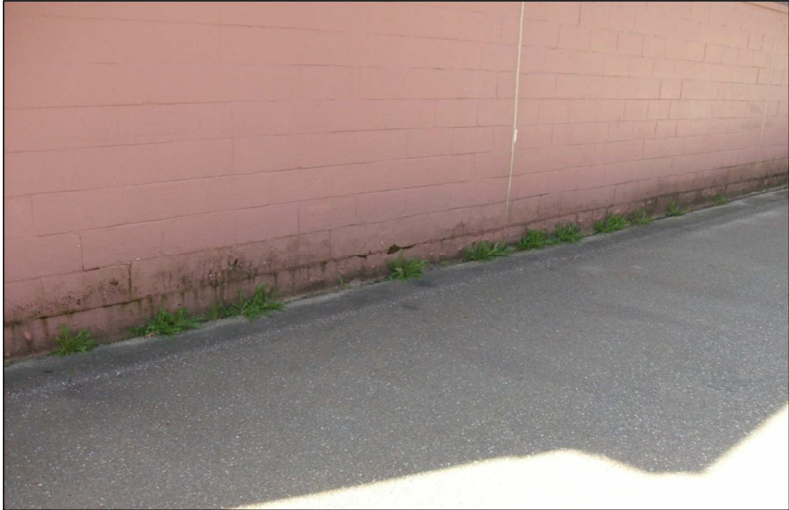
Mold/mildew growth on north side of gymnasium from roof runoff splash back.
