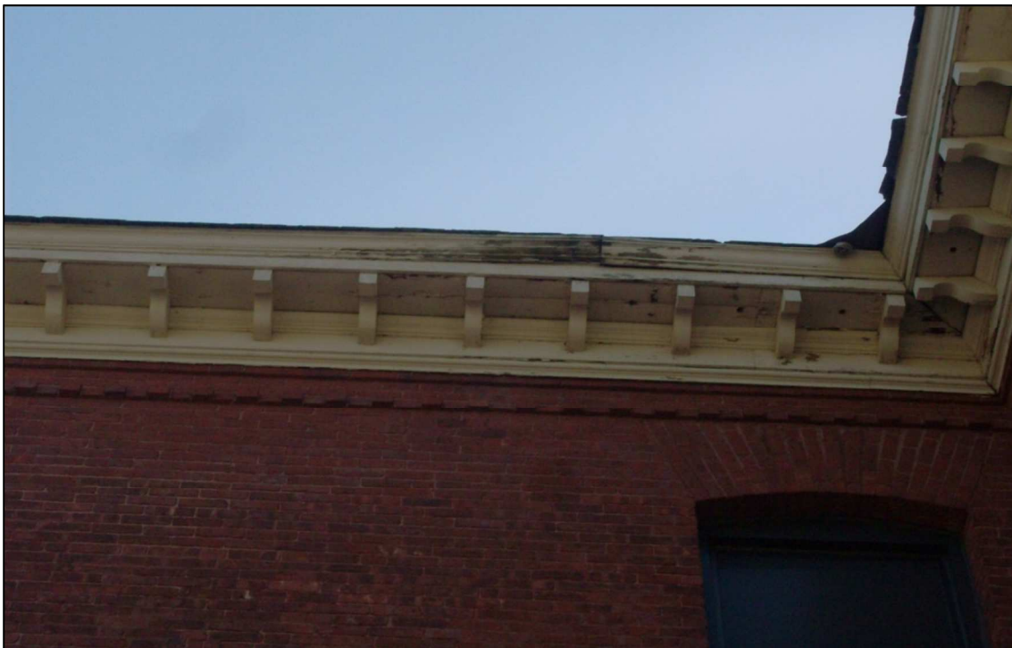
Section of rotted wood millwork at eave of original building.
