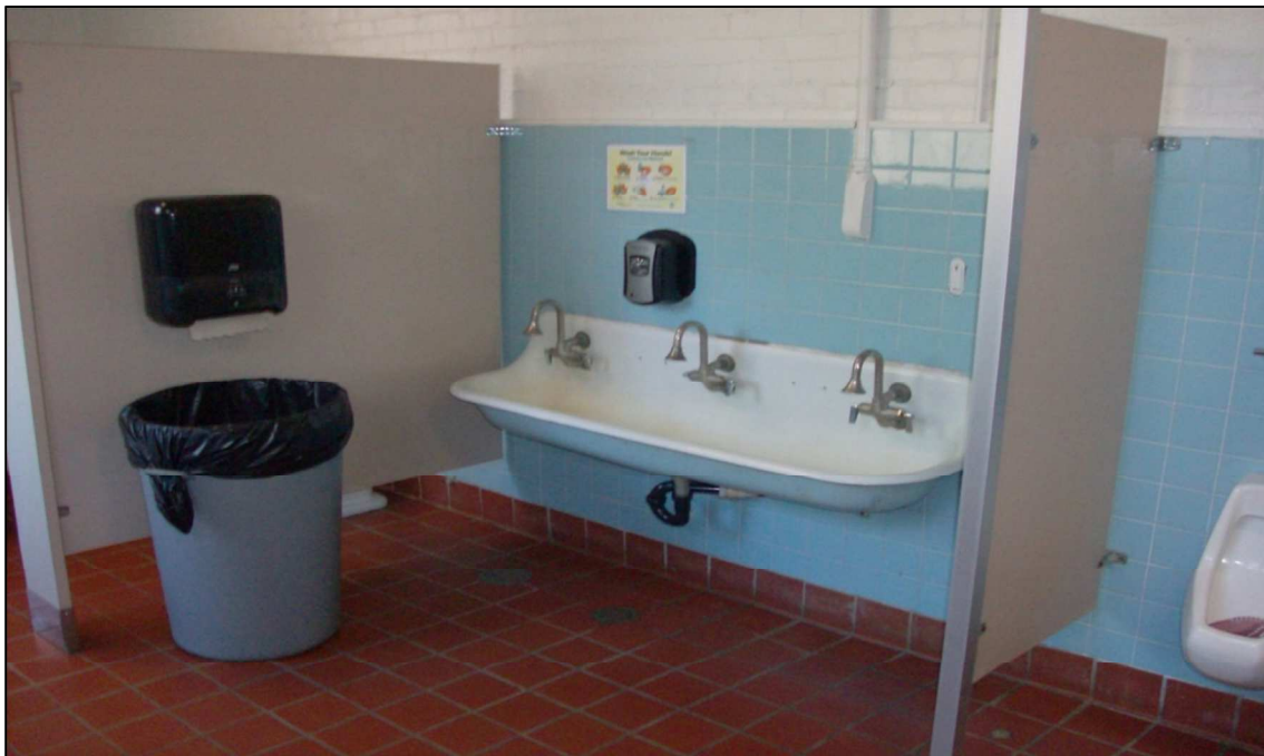
Outdated fixtures and finishes in lower level boy's bathroom.
