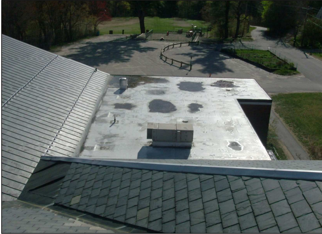
Looking east from original building toward the 1970's addition. Note metal edging along slate roof, water ponding on 1970's TPO roof, and metal roofing with snow guards on gym to the left.
