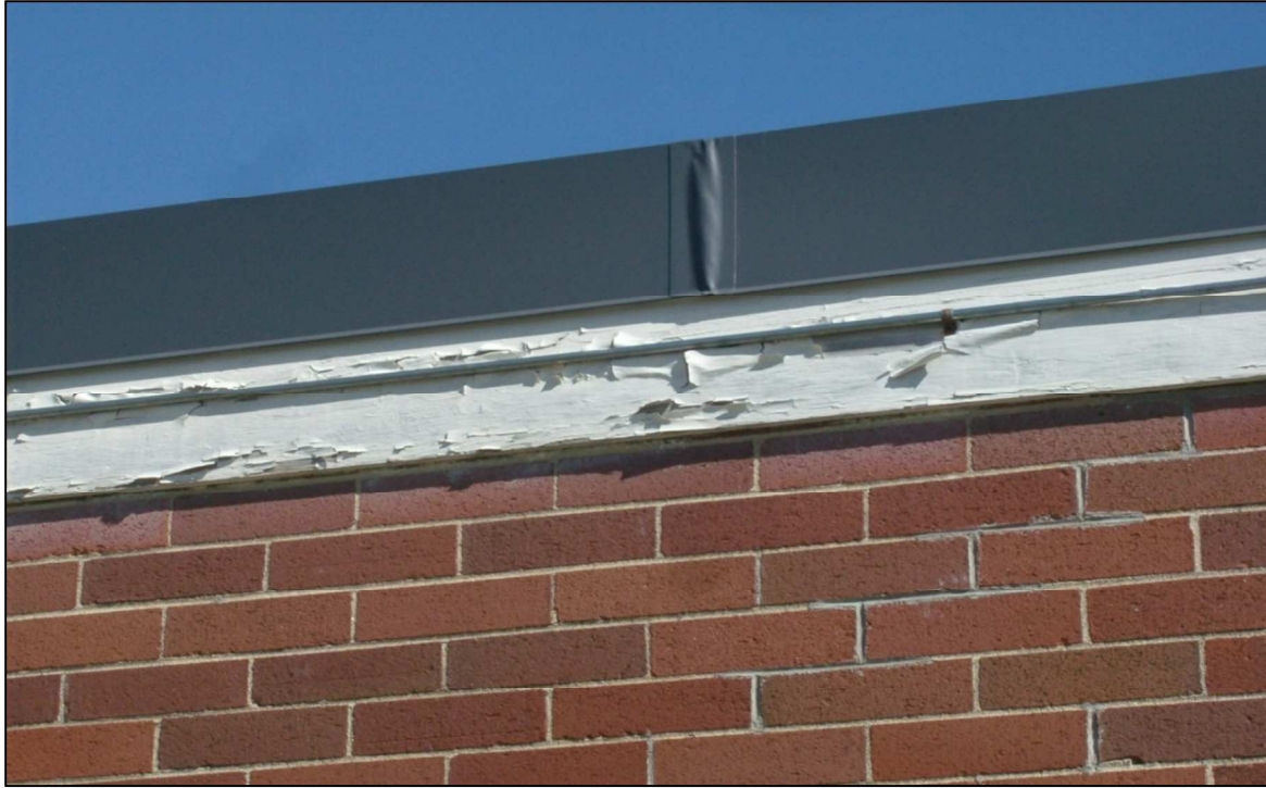
Peeling paint on wood trim at 70's addition.
