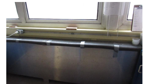
Corridor Heating Element with Foam Protection
