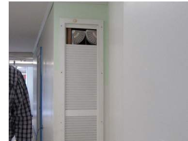
Unprotected Corridor Opening
